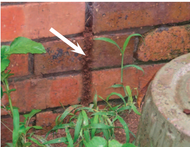
Termite mud shelter tube
